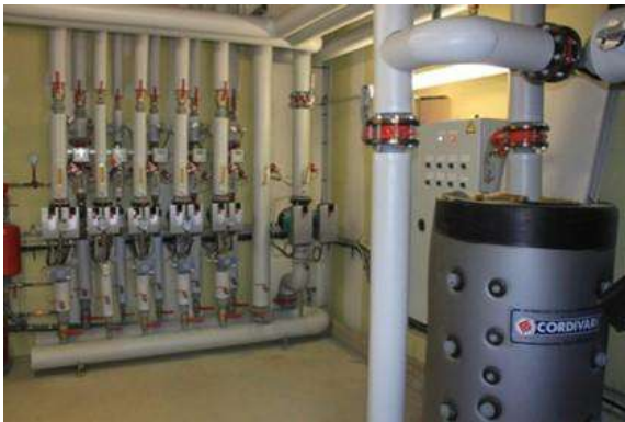
Fig. 3. Technical room (MORBIHAN ENERGIES).
